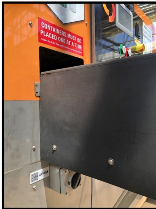
Figure 9. Power Isolator Location
