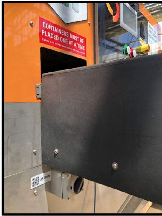
Figure 9. Power Isolator Location
