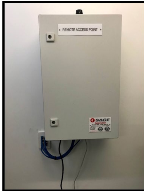
Figure 80. Remote Access Point
