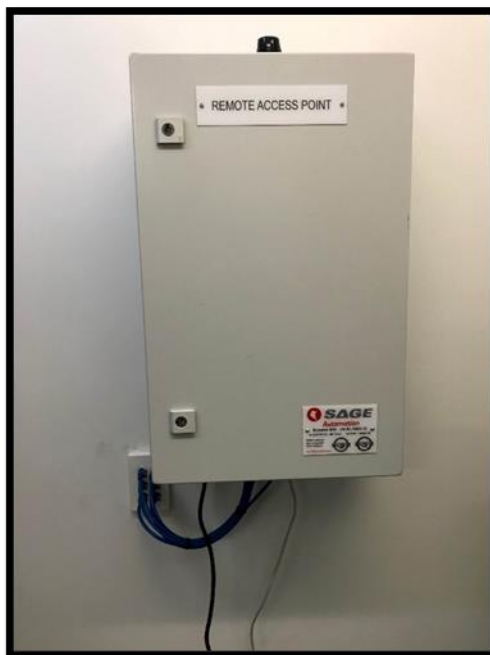
Figure 87. Remote Access Point
