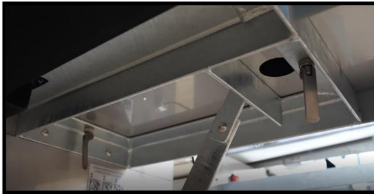
Figure 62. Unlocked conveyor cover clamping levers
