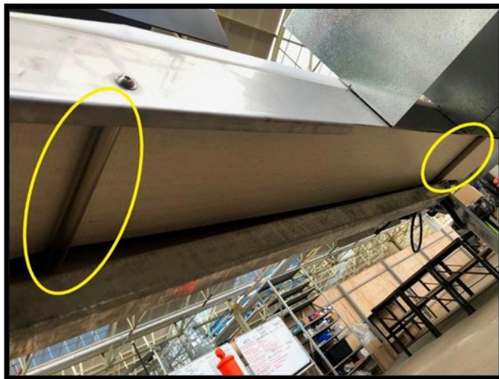
Figure 68. Underside of the belt
