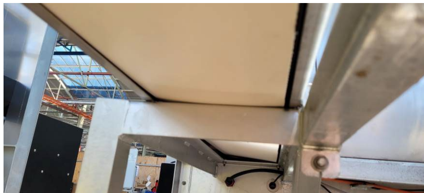
Figure 74. Incorrect belt tension
