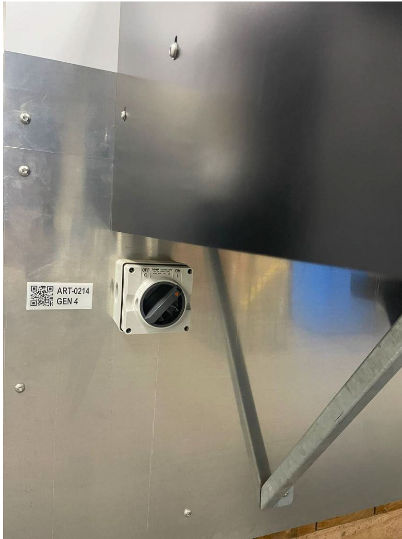
Figure 10. Power Isolator Location
